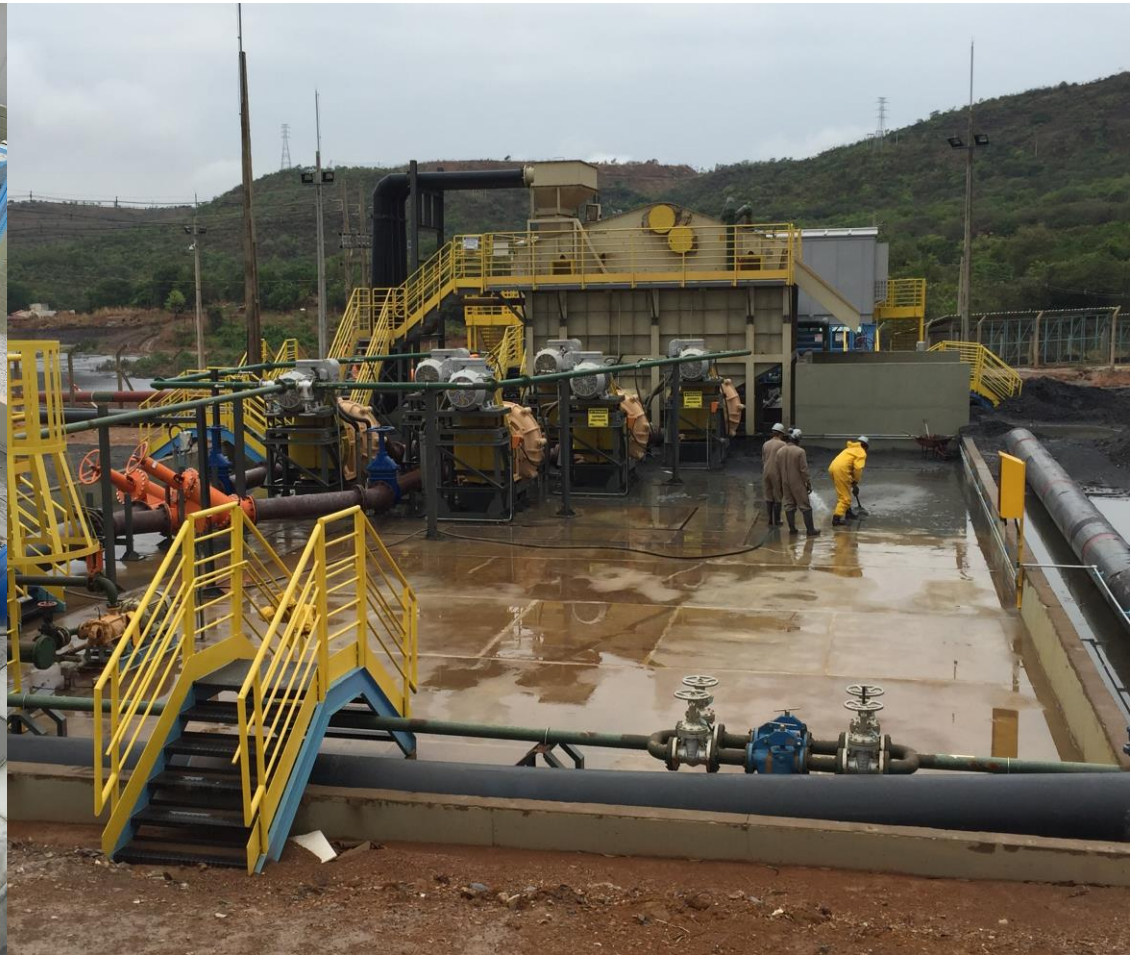
Vibrating Screen And Transfer Pumps
