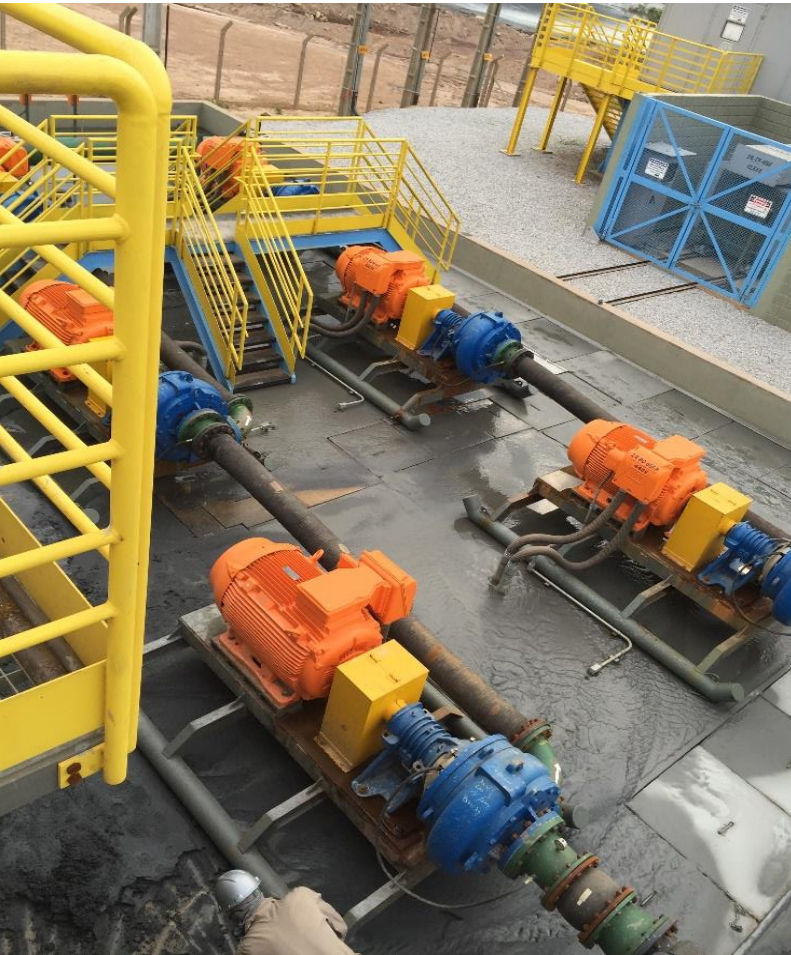
High Pressure Water Pumps
