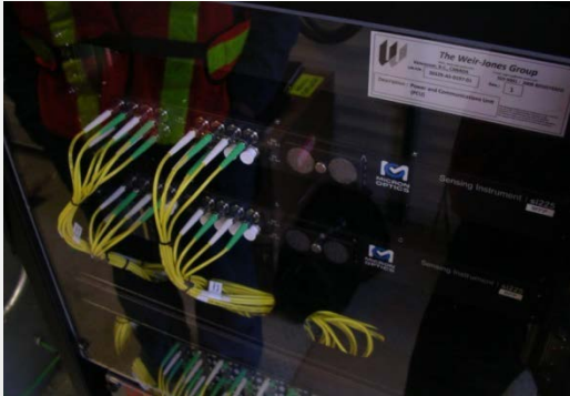
Optical Interrogator unit performing structural integrity monitoring in Northern Canada.
