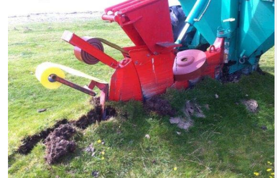
Ploughing optical fibre and warning tape into the soil. Installation rates of between 400m and 1000m/hour.
