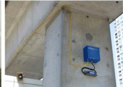
Integrity Monitoring for the Skytrain in Vancouver
