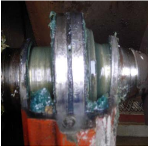
Figure 9: The grease inside the unit protected by thermoplastic polymer was clean and the bearing was in great operational condition.
