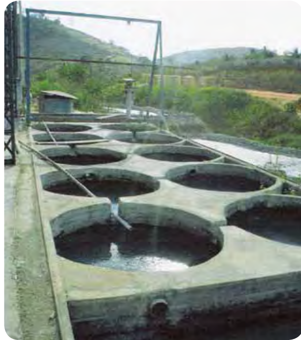
Photo 58. Effluent treatment system for waste from polishing processes. Source: Prezotti (2005)
