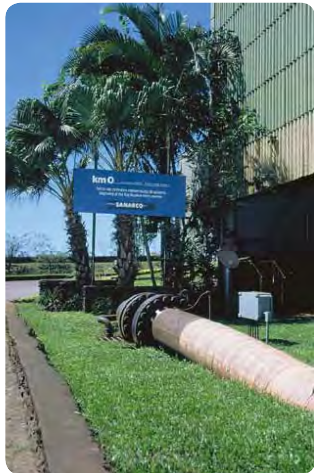
Photo 34. Ore pipeline, km 0
