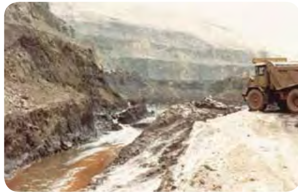
Photo 16. Trench digging for drainage and water conveyance to mine sumps. Source: MBR
