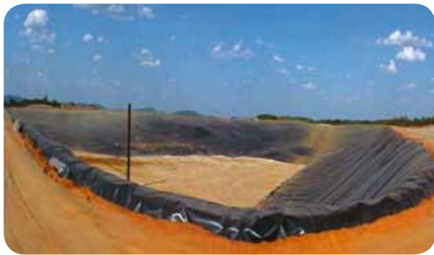
Photo 71. Overview of the dedicated tank IV
