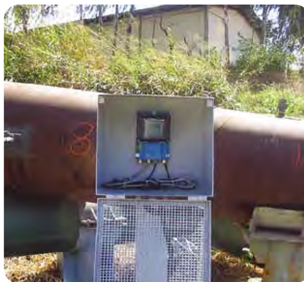
Photo 74. Flow Meter – Thirty-foot pipe
