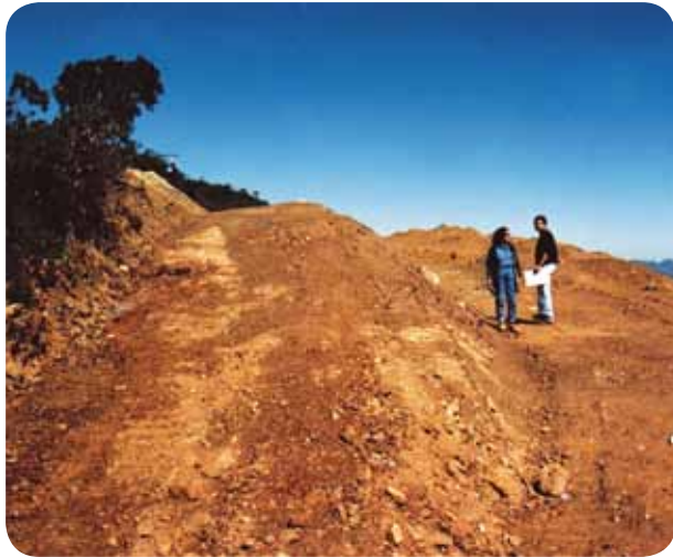
Photo 84. F2 after resloping for installation of a rainwater drainage system, followed by revegetation
