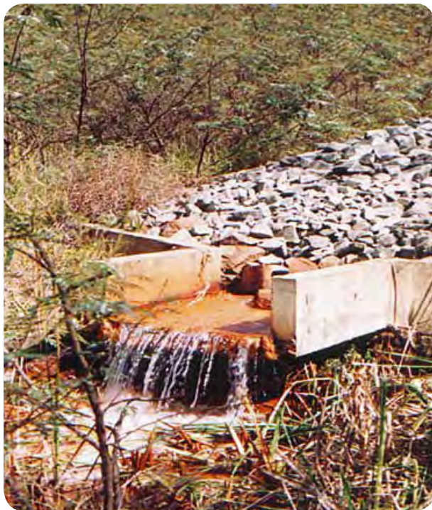
Photo 14. Water outflow through internal drainage of a dump. Source: MBR
