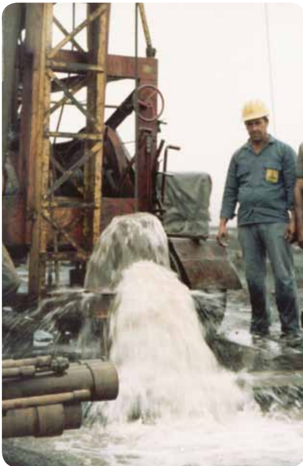
Photo 15. Underground water pumping through a deep tubular well. Source: MBR
