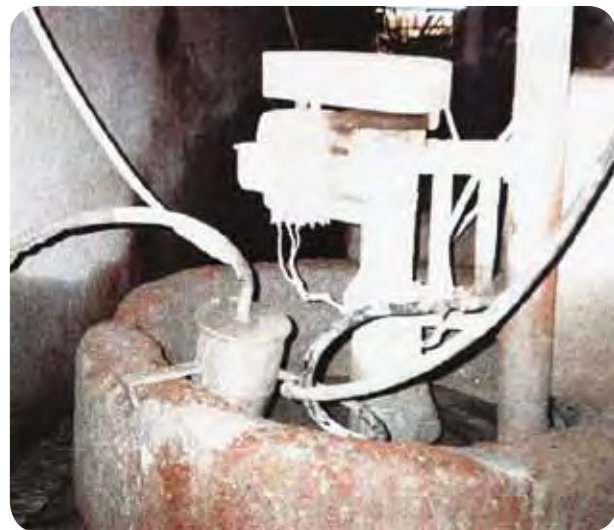
Photo 54. An abrasive sludge pumping tank; the disposal of a portion of the abrasive sludge along a collection gutter
