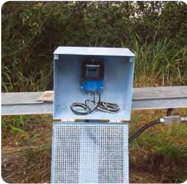
Photo 75. Flow Meter – Twenty-foot pipe
